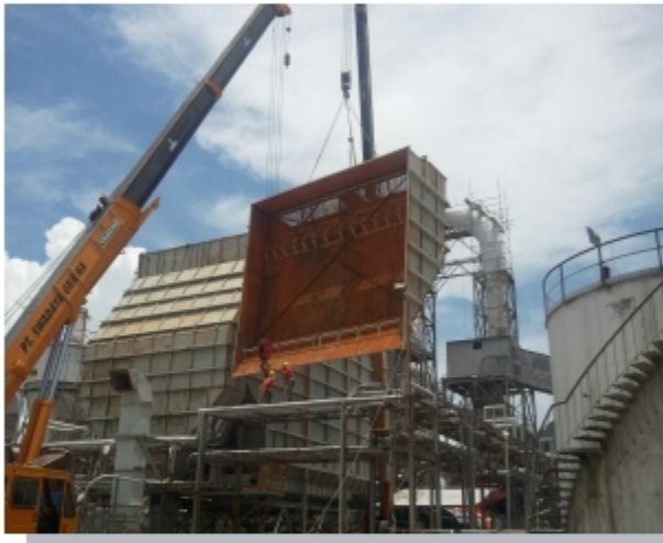
ESP Fabrication & Installation
